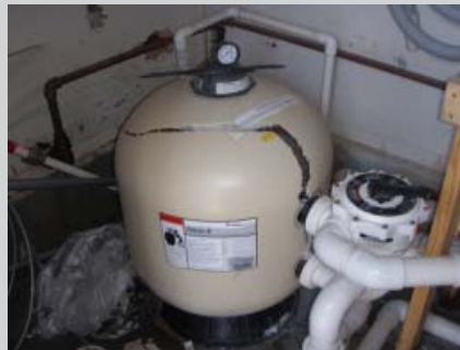
The above pool was not winterized properly resulting in a cracked filter tank and plumbing lines.
