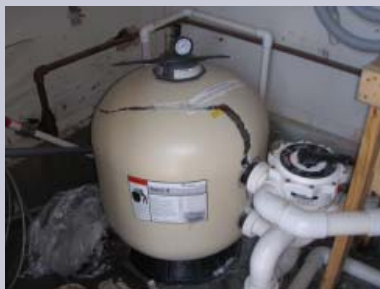
Pool was not winterized properly resulting in a cracked filter tank and plumbing lines.
