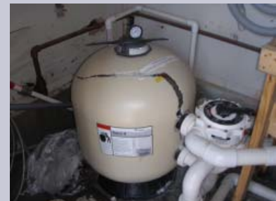
Pool was not winterized properly resulting in a cracked filter tank and plumbing lines.
